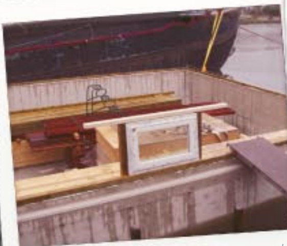
The first window's in place. It'll be followed by more than 20 others, so that it's nice and bright inside.
