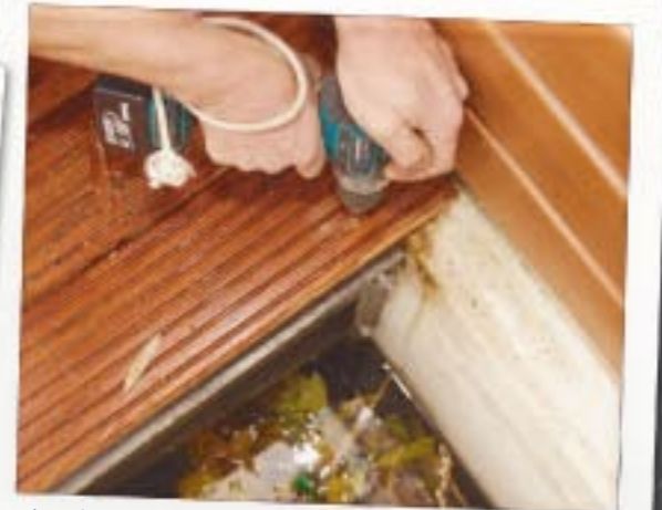
It's only outside that the water's dangerous now. I use a wrist strap to make sure the power screwdriver doesn't follow my cell phone - better to be on the safe side.
