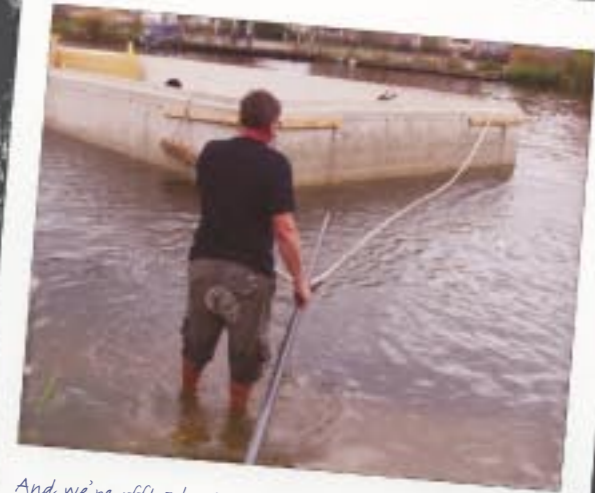
And we're off! The floating foundation for the new houseboat has arrived.
