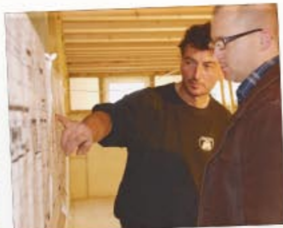
The houseboat should have absolutely everything. We discuss the sanitary system with Rob Kniesmeyer from HORNBAACH.
